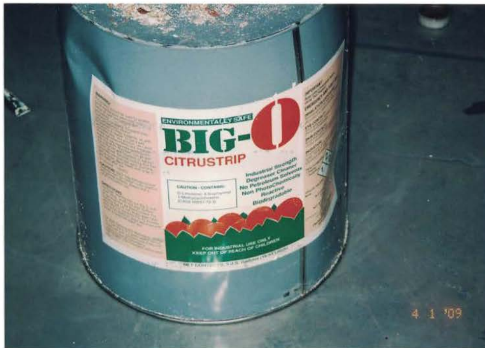
Photo #26: Spray used BIG-O CITRUSTRIP to remove asbestos-containing black mastic from the concrete floors. Note the thoroughness of the mastic removal on the recently stripped concrete floor beneath the industrial strength solvent. Viewing down.
