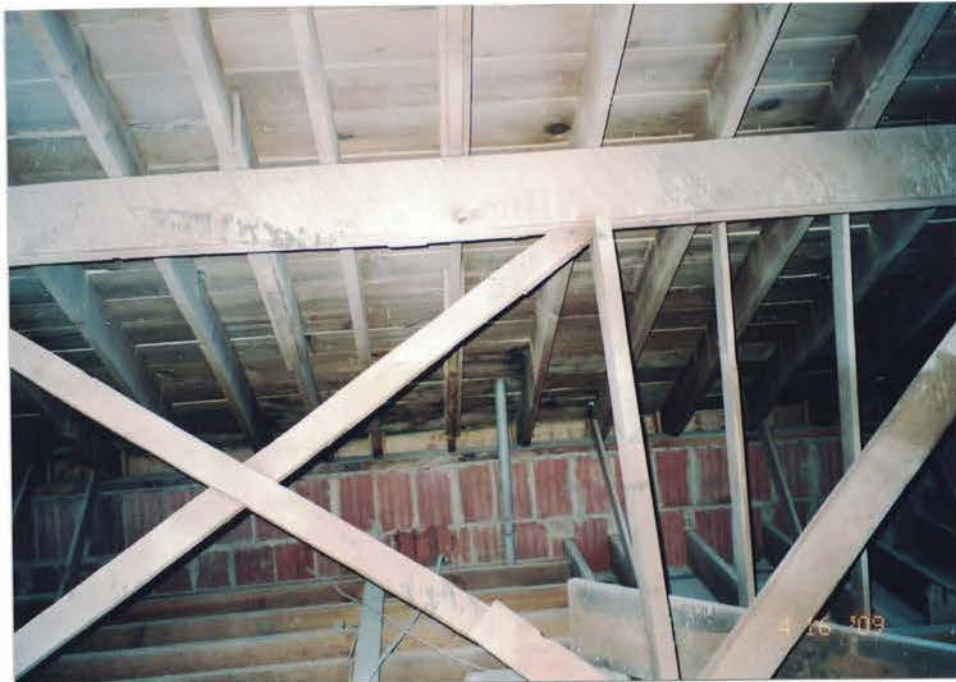
Photo #44: Spray workers scraped bat guano off the attic trusses and framing, biocleaned, and applied a light layer of encapsulant. Water stains are visible on a section of the attic trusses beneath the encapsulant. Viewing south.
