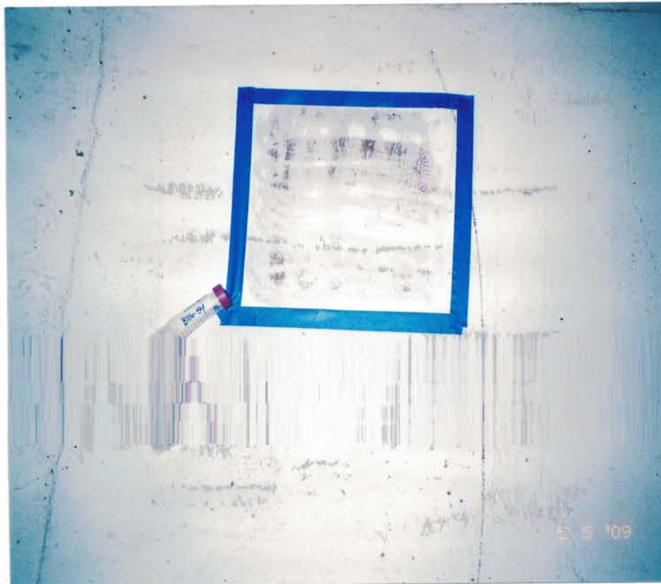
Photo #57: Post-abatement wipe sample B116-54, collected from the basement laundry room floor, is reported with a total lead count of 180 ug/ft 2 of leaded dust which is elevated, and warrants additional cleaning by Spray. Note the visible dark red paint on the concrete after the wipe sample was collected. Viewing down.
