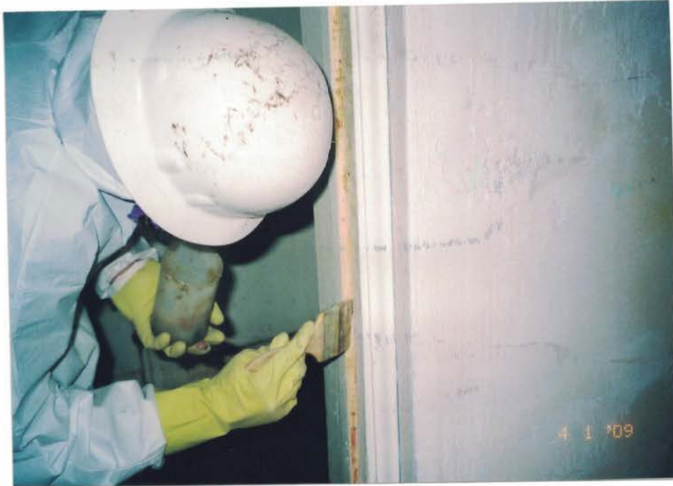
Photo #27: Spray workers apply a paint stripper to LBP on friction and impact surfaces at the location of a removed door system. Workers applied the stripper with a paint brush before manually scraping it off with a chisel. Viewing southeast.
