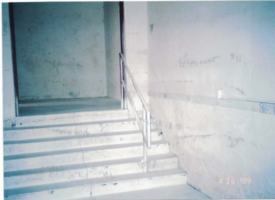
Photo #41: Spray conducted a thorough cleaning of the building by wet wiping, HEPA vacuuming, and application of a white encapsulant in order to minimize leaded dust. Note that the walls, stairs, and concrete floor inside the southwest portion of the south recreation room have been thoroughly cleaned. Viewing southwest.
