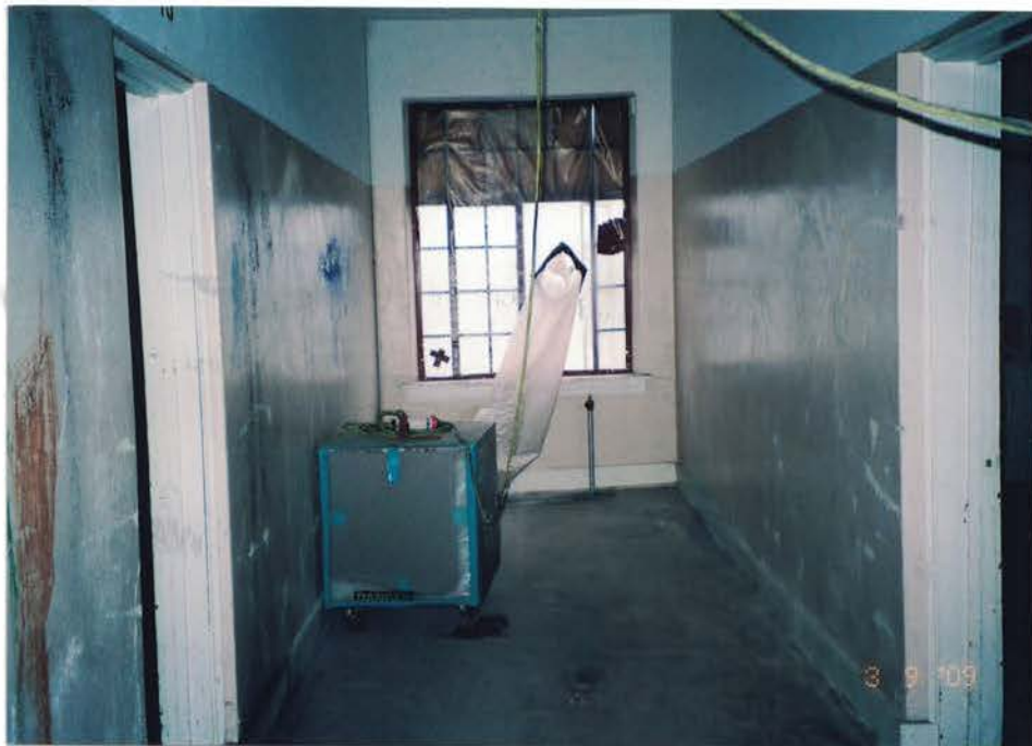
Photo #24: HEPA-filtered 2,000 cubic feet per minute (CFM) negative air machines were used during and following the abatement activities. Filtered air was exhausted to the exterior of the building through 6-mil poly tubing. Viewing east inside a side hallway.
