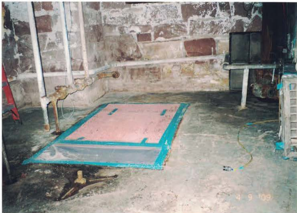
Photo #36: After removing the boiler, Spray sealed the exposed hole in the concrete floor with plywood, 6-mil poly plastic, and duct tape. Spray thoroughly cleaned the concrete slab foundation of TSI debris and soil prior to air monitoring conducted by Tallpines. Viewing northwest.
