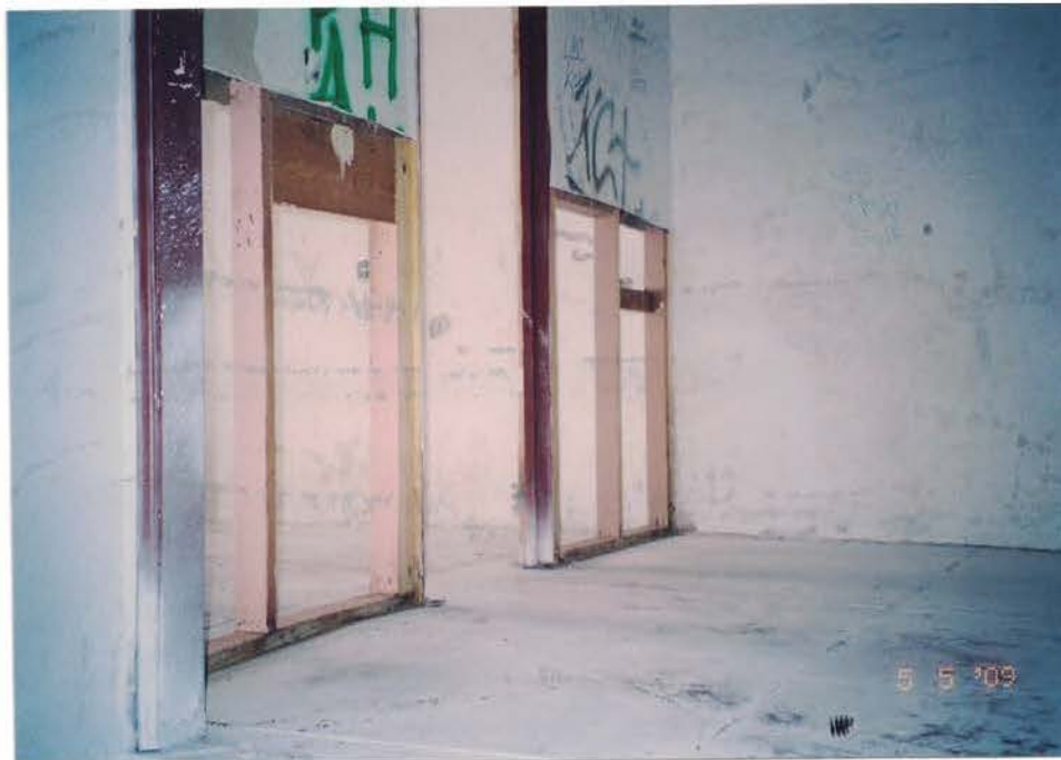
Photo #56: Inside the basement south recreation room, Spray removed mold contaminated wall systems inside the southwest rooms. Note that an approximate 4-foot height of drywall has been removed at this location. Viewing southwest.
