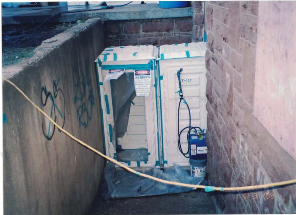
Photo #31: A three stage wet decon unit was erected at the entry to the basement boiler room. Bilingual DANGER ASBESTOS signage was posted at the entry to the regulated work area. Because the basement has a separate entry not open to the rest of the building, a separate containment was constructed. Viewing down, and to the south.
