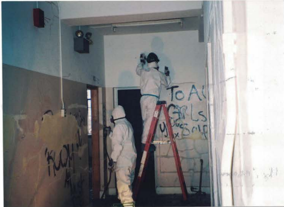
Photo #23: Spray manually scraped loose and flaking LBP to stabilize interior walls for repainting by others. Paint chips were allowed to fall to the floor before being bagged as hazardous waste. Note the Spray worker on the left spraying water into the dormitory rooms to minimize leaded dust from becoming aerosolized during the stabilization activities. Viewing northwest.
