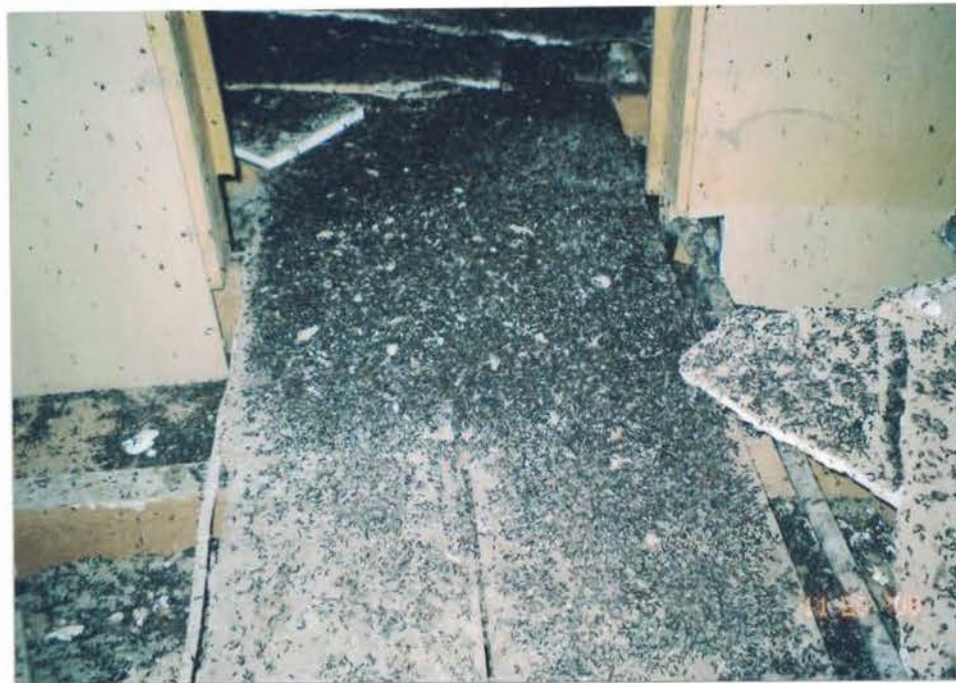
Photo #4: Copious amounts of rodent droppings cover the entire attic floor, and are up to 6-inches deep in some locations. Drywall debris, construction debris, and fiberglass insulation inside the attic have to be bagged and removed prior to biocleaning. Viewing down, and to the north.
