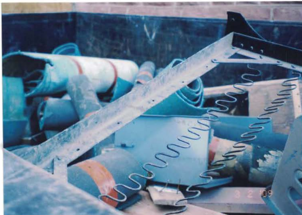
Photo #12: General construction debris, carpet, furnishings, and trash were loaded out of the building prior to the removal of hazards, and disposed of as nonhazardous waste into 40-yard waste bins located at the site. Viewing down.
