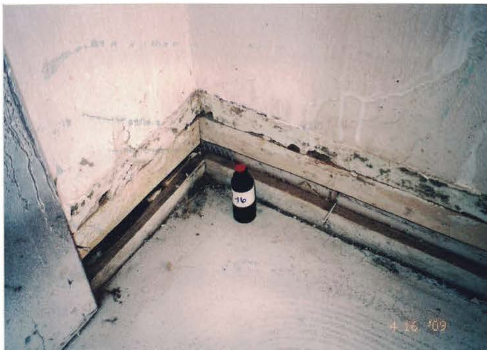
Photo #46: Post-remediation dust sample 09TEC104-16, collected inside the 1st floor Room M-1 north closet, is reported with 0.49 mg/g of mouse allergens. Droppings are still inside the wall cavities, but based on the analytical test results, do not represent a current hazard. Viewing down, and to the northwest.
