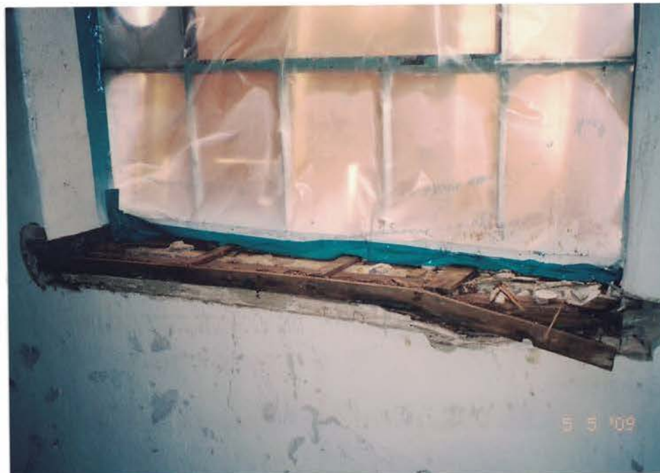
Photo #58: A LBP window sill inside the basement laundry room was removed for disposal as per the contract specifications. The LBP wooden sill is not historical, and warrants removal and disposal instead of stripping in-place. Viewing down, and to the southeast.
