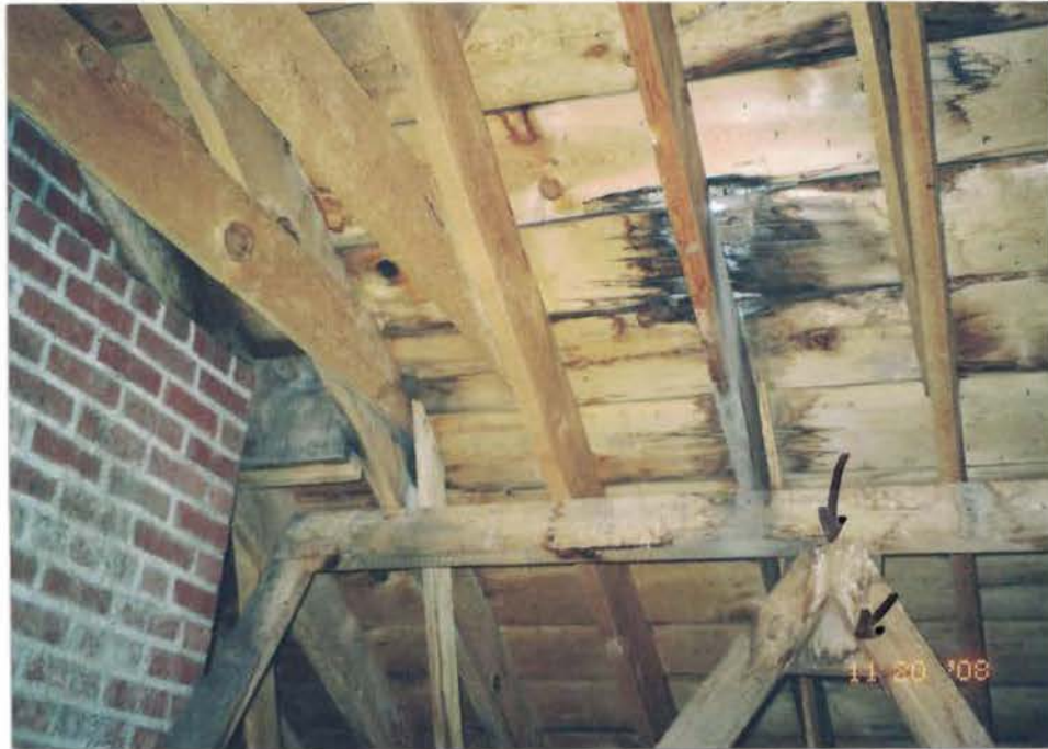
Photo #3: Water-damage from roof leaks are visible inside the attic on the wooden plank sheathing, and wooden roof trusses. White bat guano is present on roof framing (arrows), and on the attic floor. Viewing up, and to the northeast.
