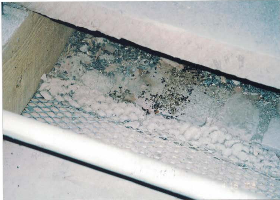
Photo #43: During the post-remediation visual inspection for biohazards, Tallpines noted minor amounts of rodent droppings missed by the Spray crew. Spray workers immediately HEPA vacuumed and biocleaned this portion of the metal lath & plaster floor. Viewing down, and to the southwest.
