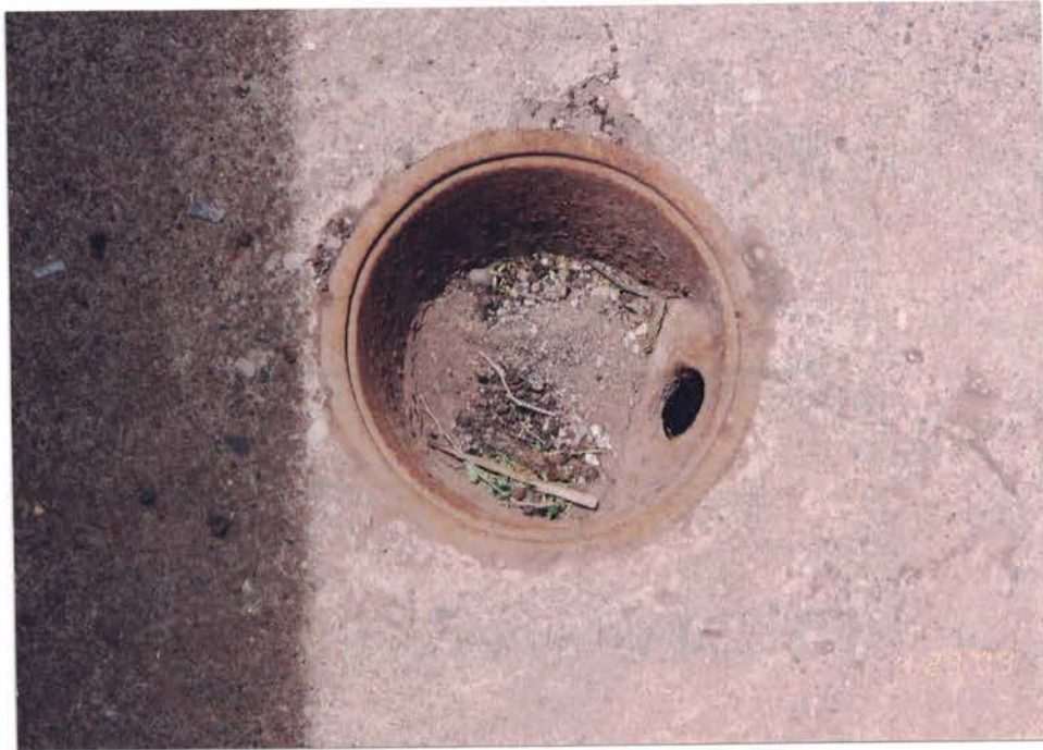
Photo #55: Stormwater debris visible inside the metal floor drain in the concrete areaway following a recent storm. Installation of wire screens, and routine maintenance of the floor drains will be mandatory to prevent future flooding in the basement. Viewing down.
