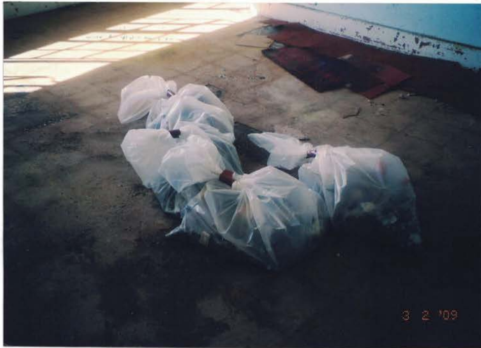
Photo #19: Bagged carpet waste, contained in 6-mil poly waste bags, was removed from the 1st and 2nd floors, and from the full-basement. Viewing down, and to the south-east.
