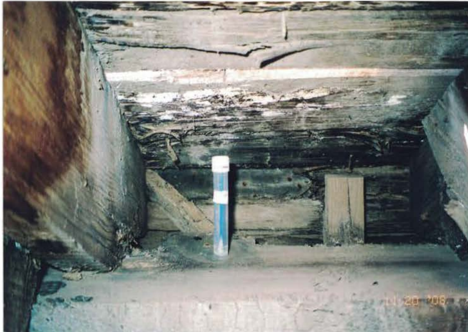
Photo #6: Inside the attic at the location of the portico roof, there is water-damage, structural damage, staining, and mold contamination. Swab sample 08TEC304-01 is reported with elevated counts of fungal mold that warrants removal of contaminated materials. Viewing west.
