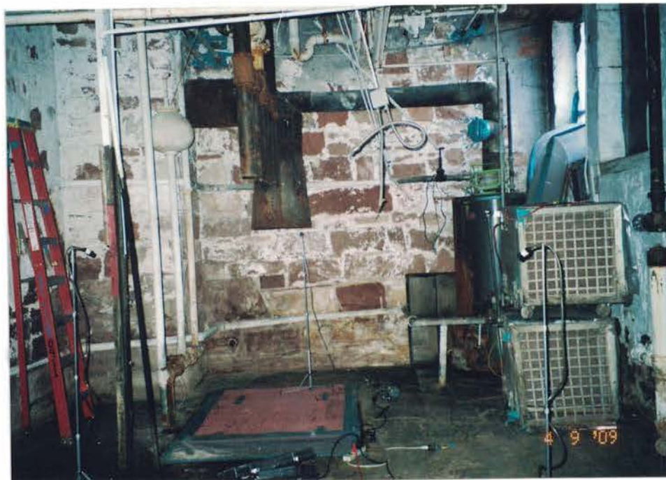
Photo #32: Post-abatement clearance air samples, collected inside the boiler room, are reported < 17 structures per square millimeter ( \text{str}/\text{mm}^2 ) of asbestos which is well below the AHERA clearance standard of < 70 \text{str}/\text{mm}^2 . Following the stripping of TSI, the boiler was removed for recycling of the metal. Compare this to photograph #9. Viewing north.
