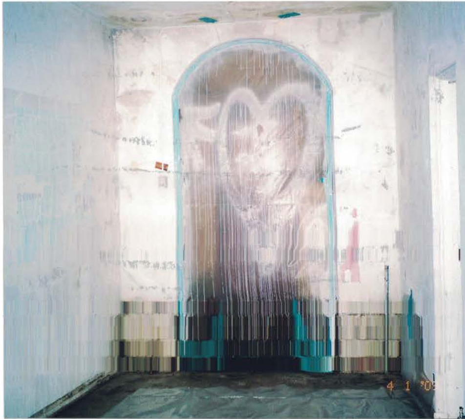
Photo #29: Spray applied 6-mil critical barriers over the main entry to the building. A white encapsulant paint was applied to the wall systems after loose and flaking LBP paint was manually scraped off the walls. Spray bagged the LBP debris and used a HEPA vacuum to clean before washing and encapsulating the walls. Viewing west.
