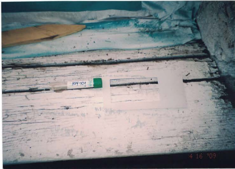
Photo #47: One of hazards removed by Spray from Building 116 was mold. Post-remediation swab sample 09TEC104-01, collected from the 2nd floor Room 2-7 west window sill, is reported with a nonelevated count of fungal mold. Viewing down, and to the west.
