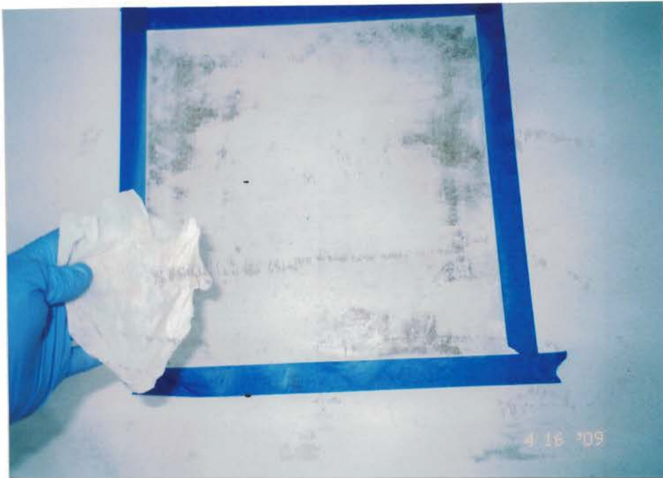
Photo #39: Post-abatement wipe sample B116-14, collected from the concrete floor inside 1st floor Room M-4, is reported with a lead content of 23 micrograms per square foot ( \text{ug}/\text{ft}^2 ) which is below the HUD clearance standard of 40 \text{ ug}/\text{ft}^2 for floors. Viewing down.
