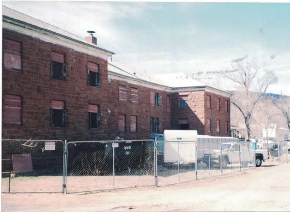
Photo #11: Spray erected a temporary chain-link fence around the building for the duration of the abatement of hazards. The entire building became the regulated work area (requires a respirator and protective clothing to enter). Viewing northwest.
