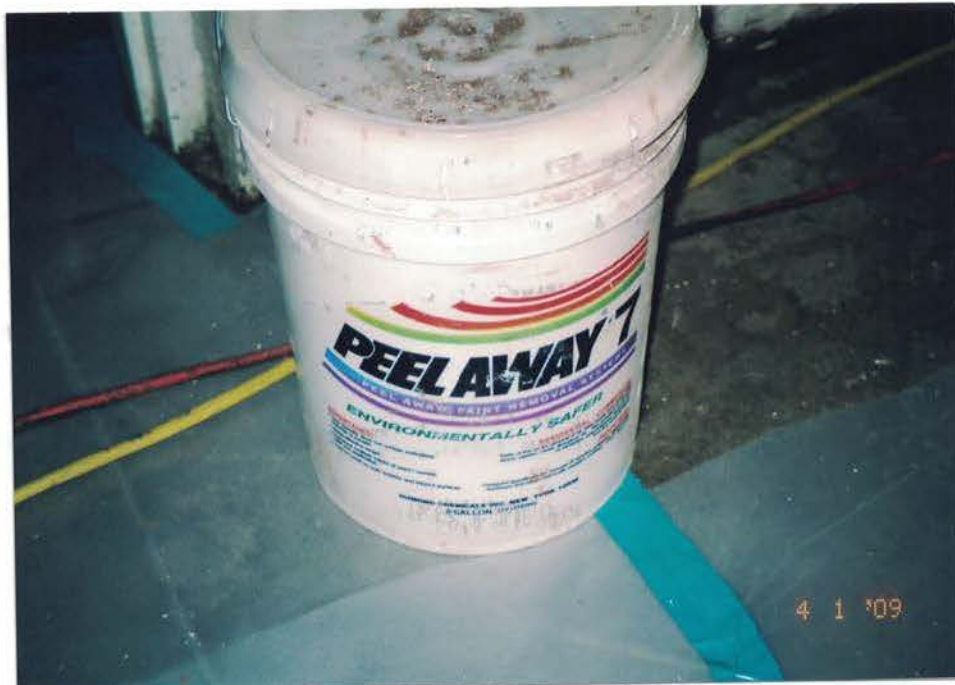
Photo #28: Spray used PEEL AWAY 7, a paint remover, on friction and impact surfaces before scraping off the paint. Viewing down.
